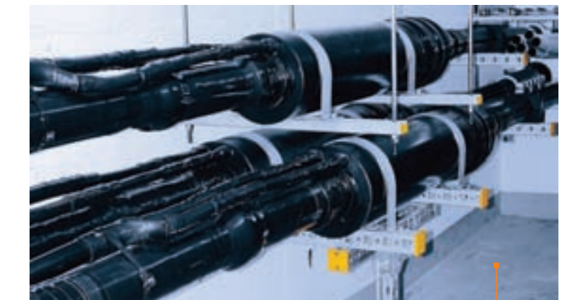
Laying in a tunnel: Joints with Cu-tube and HDPE-coating in a tunnel.
